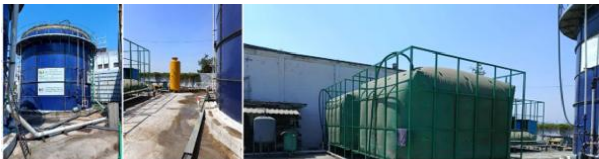
Image 5: Bowenpally's Biogas Plant
