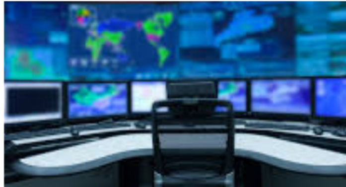
Command and control centers
