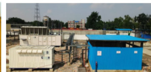
View of Hydrogen Facility
