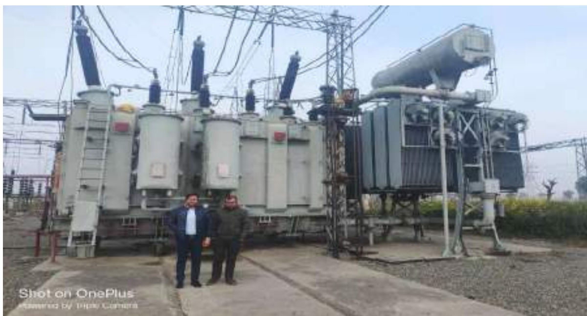
PSTCL Substation of 220KV at Baghapurana, Moga
