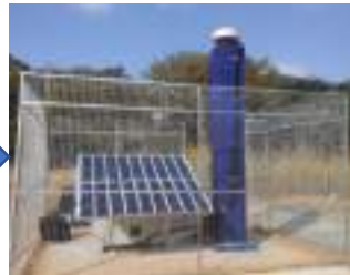
CORS Station Setup
