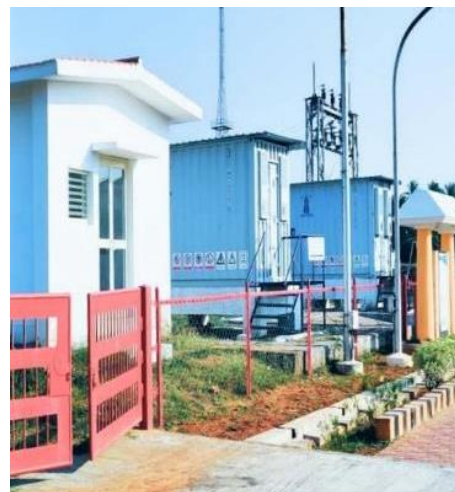
Battery energy storage (Photo Credit: USAID)
