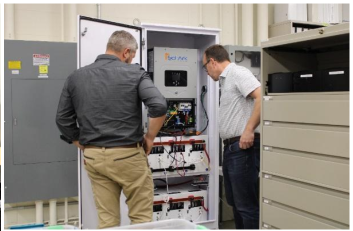
Battery and controller installed at WSU Pullaman to provide battery backup of key systems during an outage. BESS supplied by Larsen & Toubro. (Photo Credit: Department of Energy)
